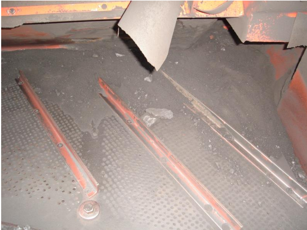
Figure 4: FGX table deck blocked by damp fine coal
