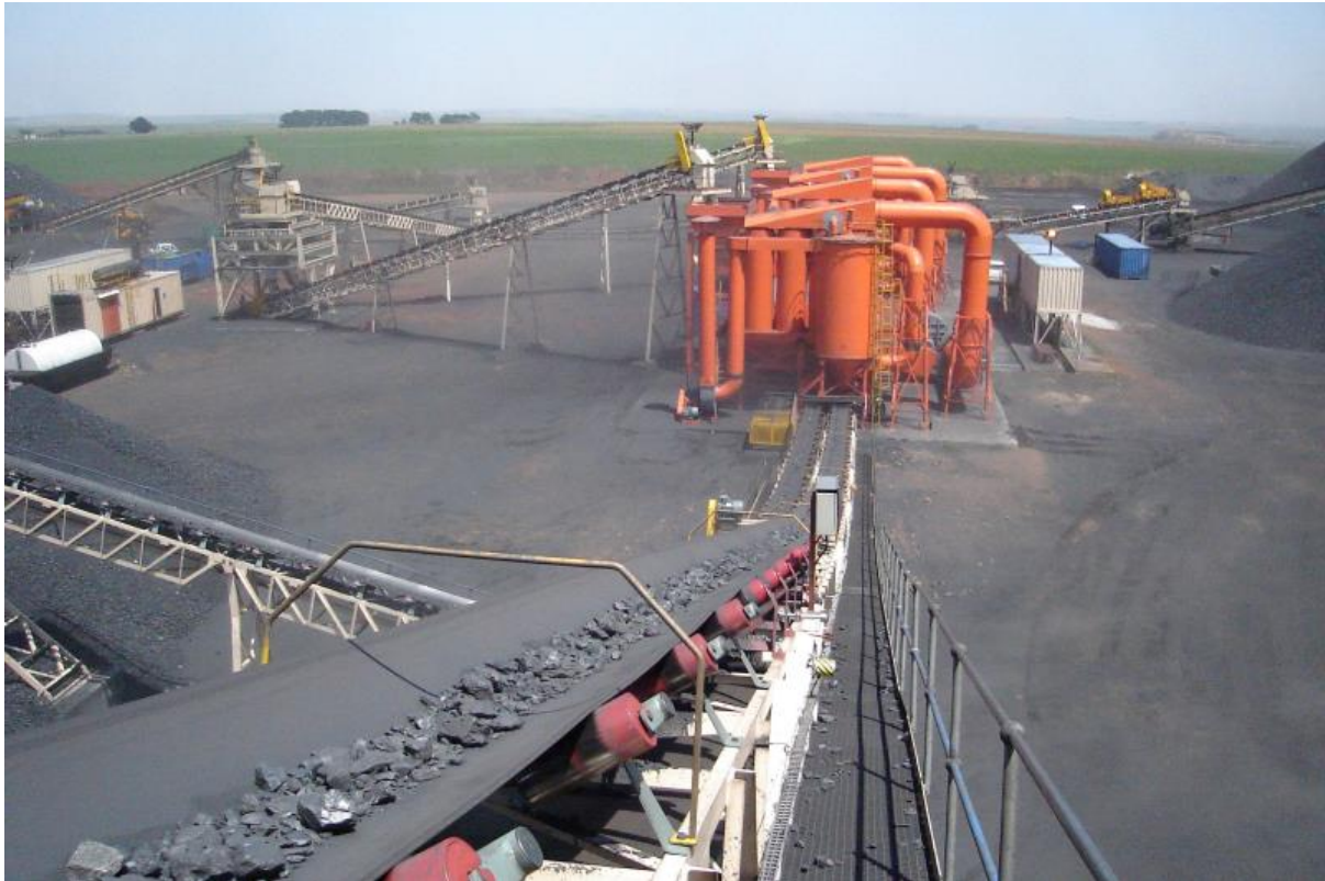
Figure 5: FGX plant at Middelkraal
